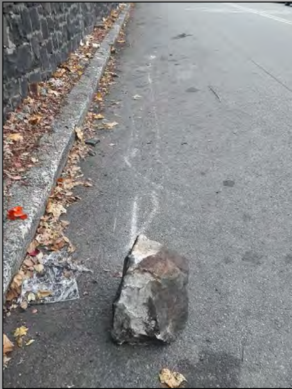
Loose Stone that fell onto Roadway
